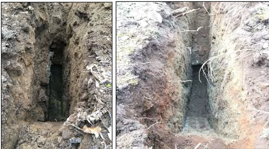
Photo 4 & 5: Subsurface Conditions at TP-1 (left) with roughly 5.5 feet of uncontrolled fill and TP-7(right) depicting native soil conditions as observed across the majority of the project site.
